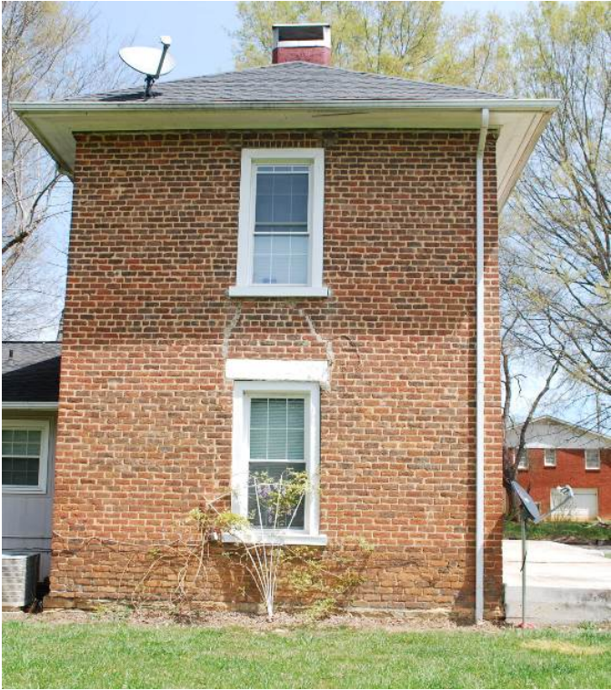
Photograph 7. West Elevation and Structural Cracking
